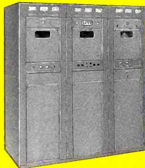
BC-5P-2 5 KW AM Transmitter
